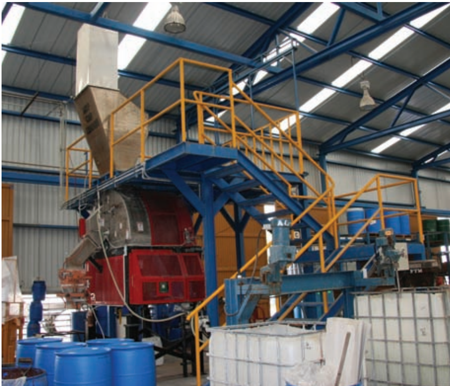
The platform, which is built around the mixer, holds three fully loaded pallets of powder ingredients and allows an operator easy access the mixer's dust-free bag-dump station.
